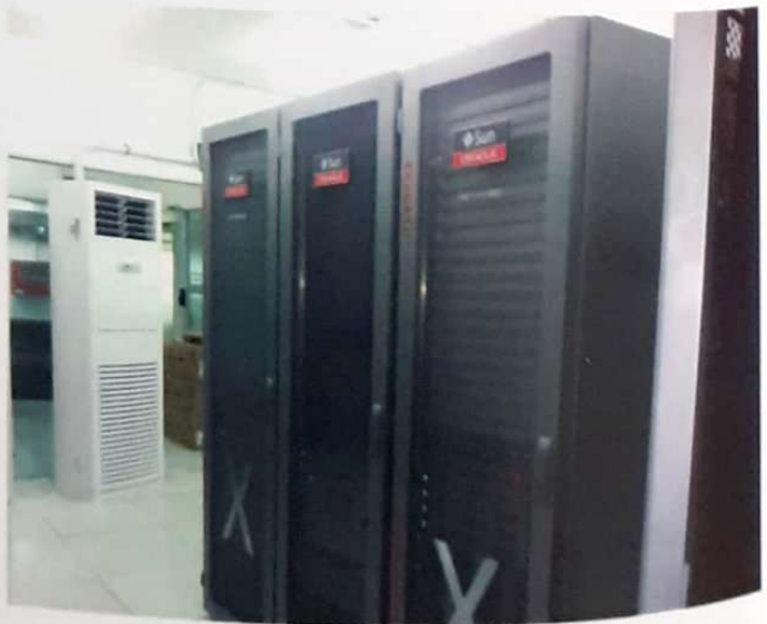
Pubali Bank has Built a robust Data Center.
